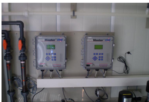
New cooling water control device
